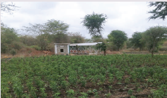
The Solar pump system installed by I&M Foundation
